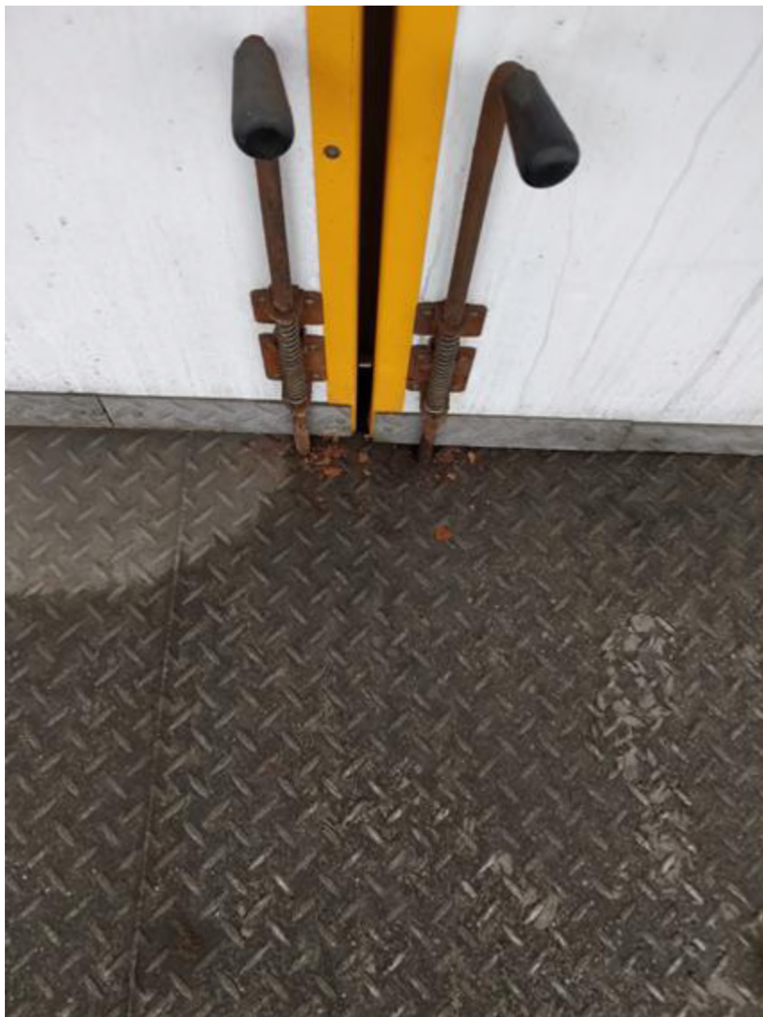
Fig. 5. Corrosion of internal fittings
