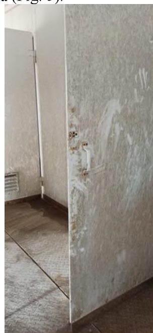
Fig. 4. Corrosion of paint coating of doors and walls
