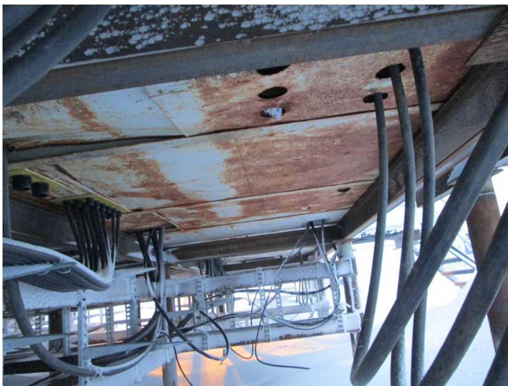
Fig. 2. Corrosion destruction field of object 2
